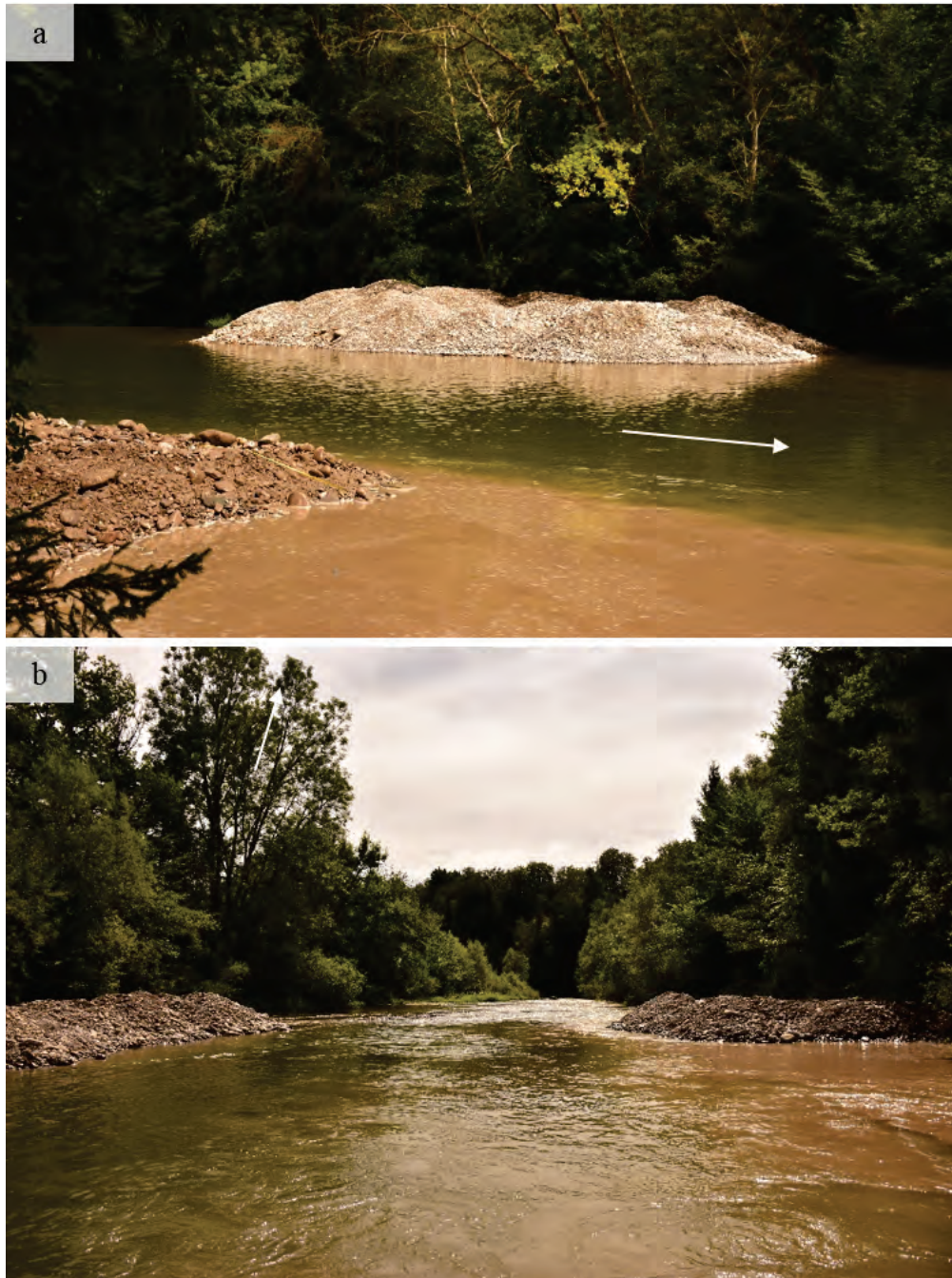
Figure 9.4 – (a) View on the most upstream deposit placed on the left bank, (b) third and fourth deposits placed on the banks, (c) first and third deposits viewed from downstream, (d) machine operating the sediment replenishment placement
